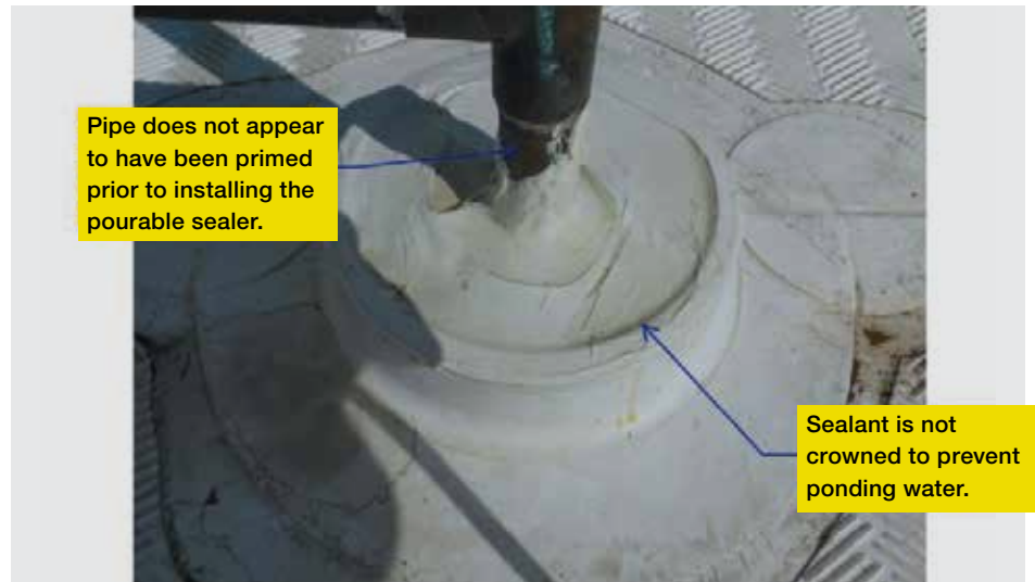
Figure 8. Example of incorrectly installed sealant - pocket flashing. The sealant in the pan is not crowned, and the contractor did not prime the thermoplastic olefin membrane flashing or the pipe before installing the pourable sealer.
