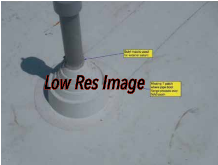
Figure 2. Example of an incorrectly installed prefabricated pipe boot penetration. The wrong sealant was used at the exposed surface against the pipe, and T patches are missing where the pipe boot flange crosses field seams.
